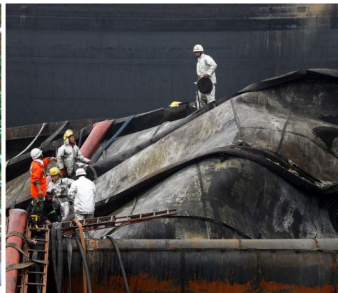
Burst pipeline, Dailan China – wireless type of corrosion?
